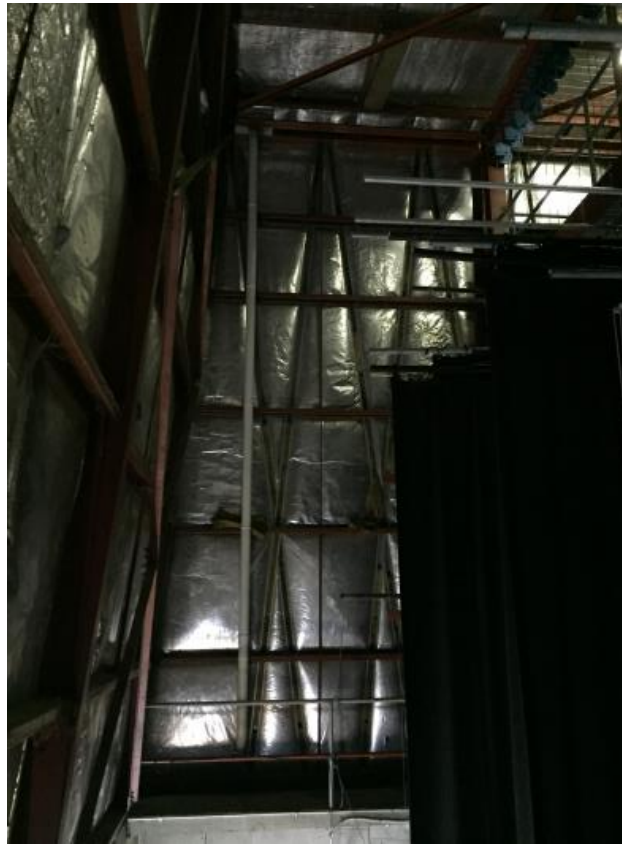
Site Photograph 11 – several penetrations through fly tower cladding, including roof drainage
