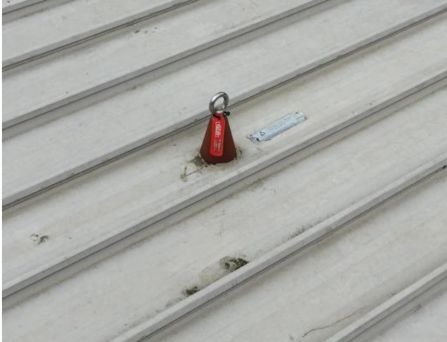
Site Photograph 15 – majority of anchor points had been recently tested and tagged “failed”
