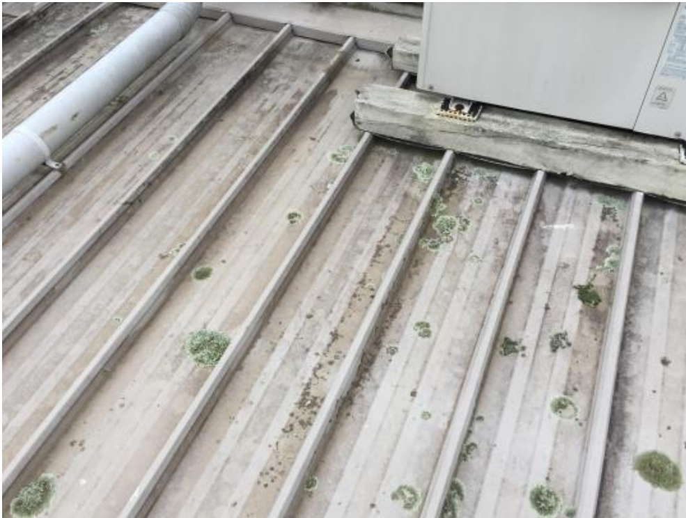
Site Photograph 19 – mould build up sighted, possibly from water ponding on roof deck (DP spreader shown top left of photograph)
