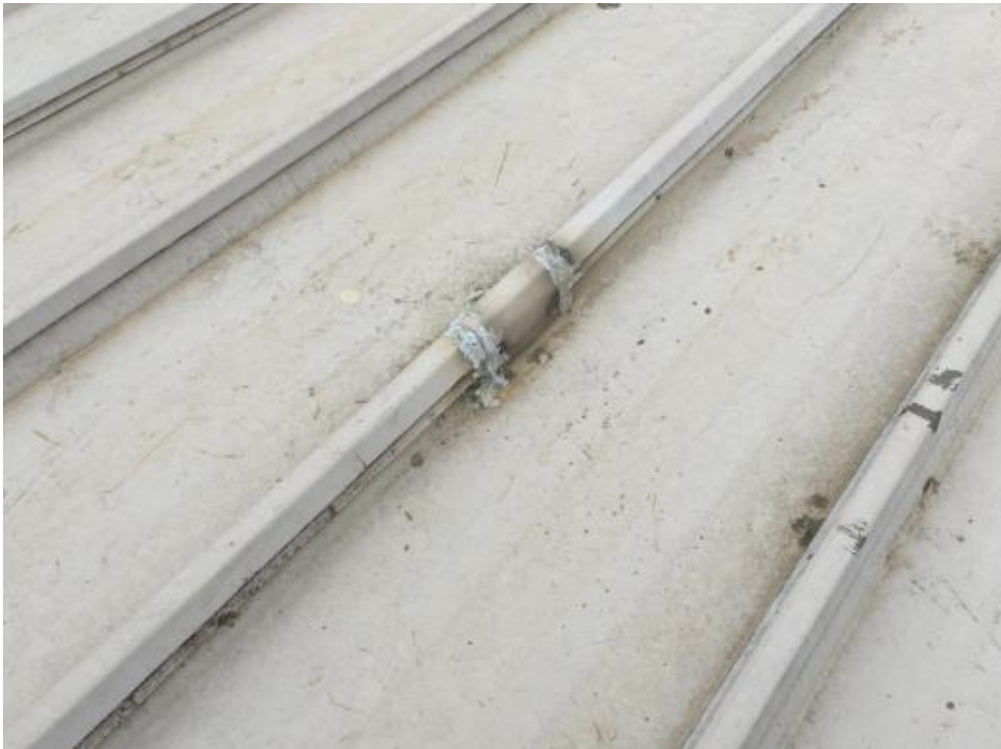
Site Photograph 21 – mould build up sighted, particularly around flashing elements
