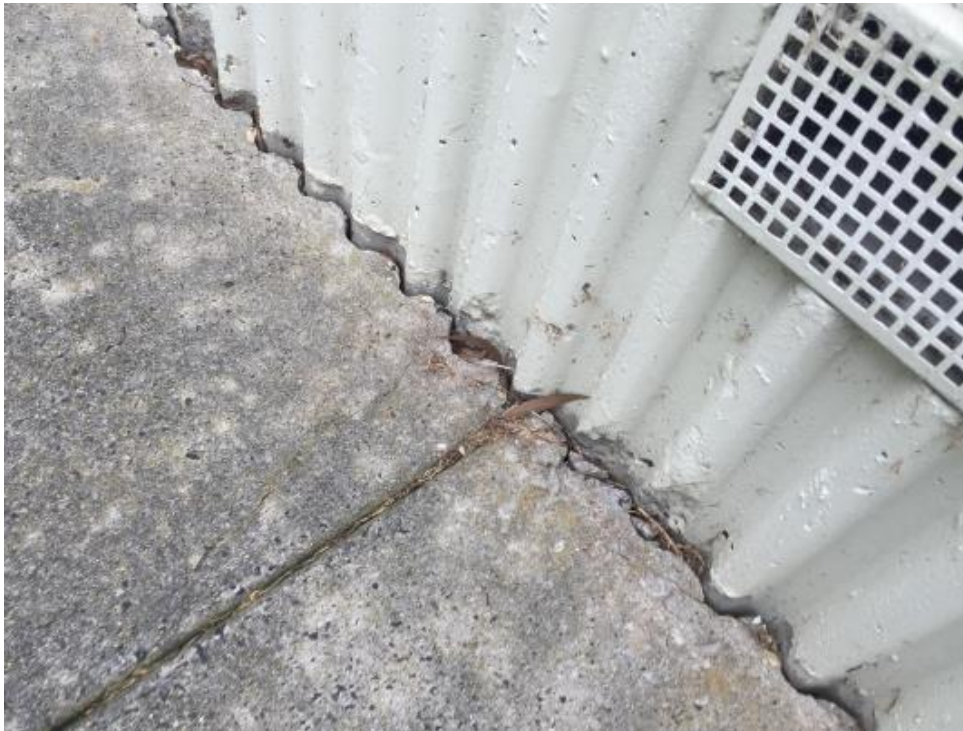
Site Photograph 7 – concrete pavement settled however building appears structurally sound
