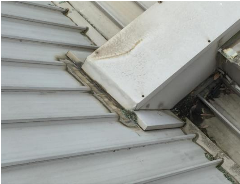
Site Photograph 23 – mould build up sighted, particularly around flashing elements
