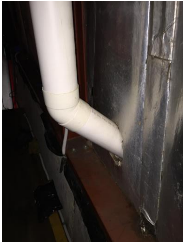
Site Photograph 9 – downpipe penetration through fly tower cladding
