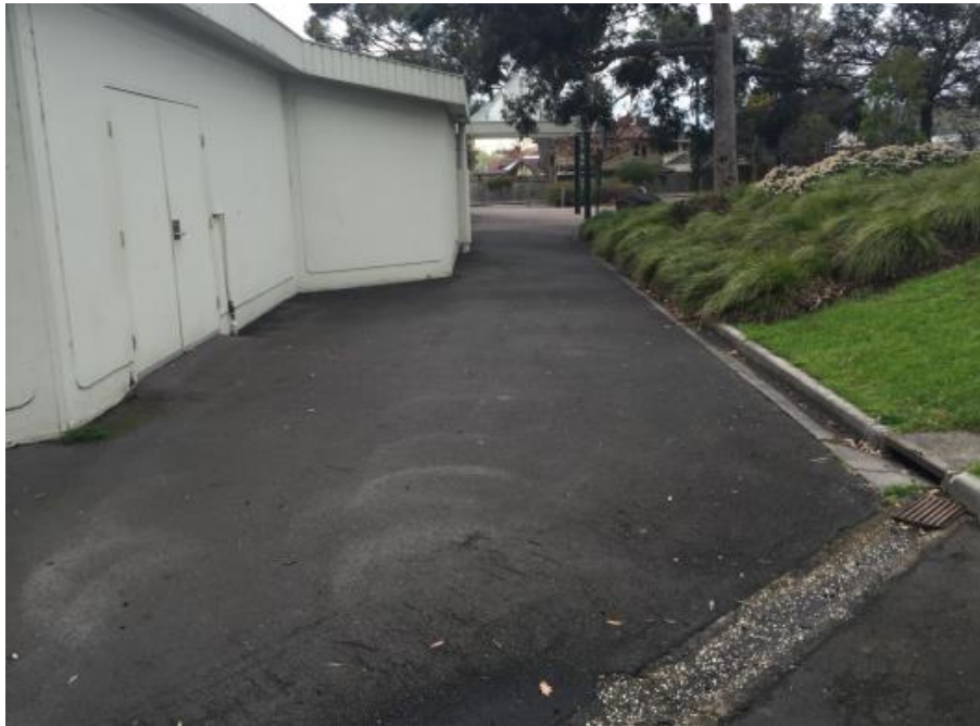
Site Photograph 3 – perimeter pavements generally fall away from building to drainage infrastructure (kerbs, pits etc.)
