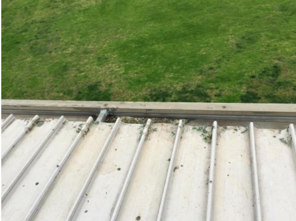
Site Photograph 17 – gutters generally appeared well maintained on inspection, appeared moisture has ponded on areas of roof sheet (mould build up)
