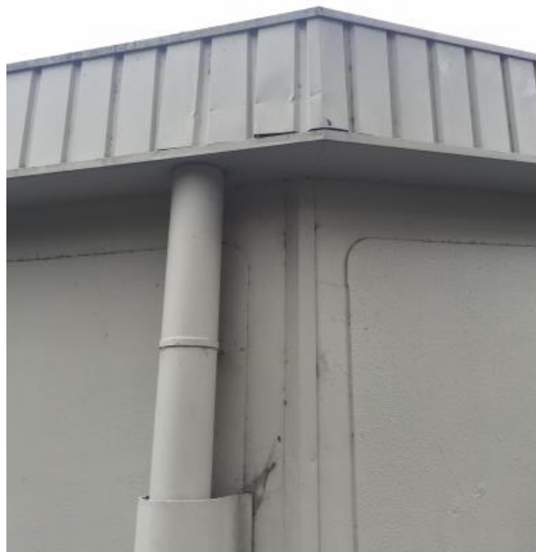
Site Photograph 1 – slight damage to gutter and external clad
