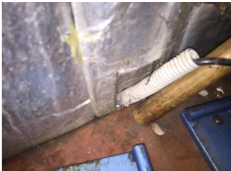
Site Photograph 12 – penetration through fly tower cladding
