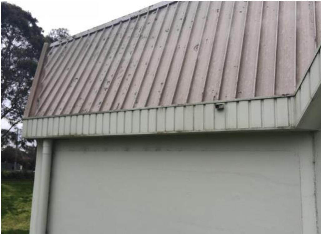
Site Photograph 5 – deterioration sighted in roof sheet
